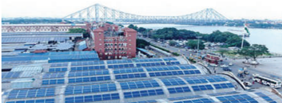
Photo: Solar panel installed at Howrah railway station
