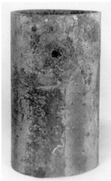
FIGURE 8.5.16 Pitting on boiler tube. (Courtesy of The Metro Group, Inc.)
