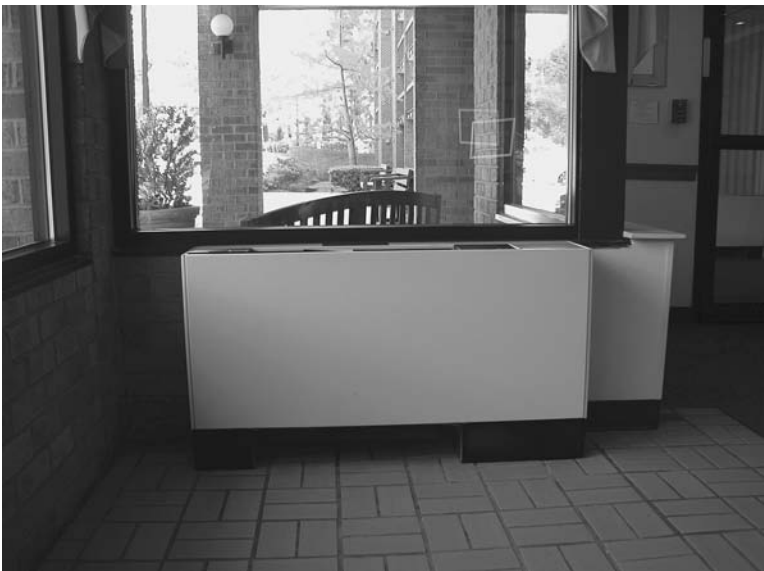
FIGURE 7-8 Photograph of a cabinet fan-coil unit.
