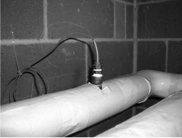
FIGURE 9-1 Photograph of a temperature sensor installed in a pipe.
