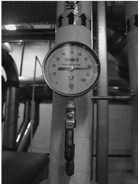
FIGURE 3-33 Photograph of a pressure gauge mounted in pipe.
