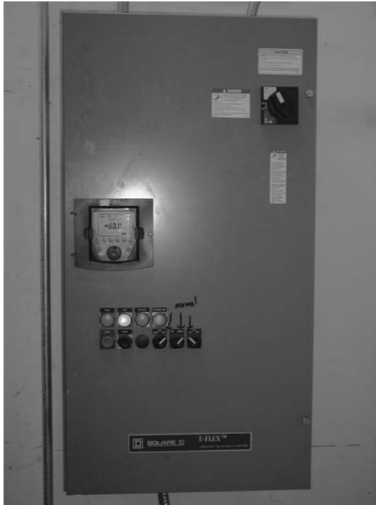
FIGURE 9-14 Photograph of a variable frequency drive with a hand-off-automatic switch and a bypass contactor.
