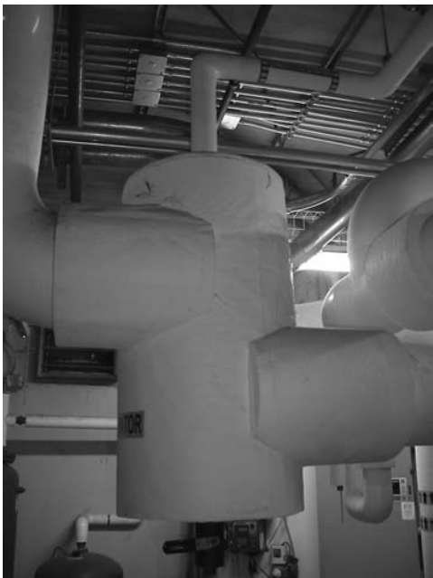
FIGURE 4-20 Photograph of an air separator.
