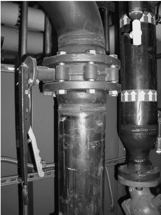
FIGURE 3-14 Photograph of a lug-style butterfly valve—installed.
