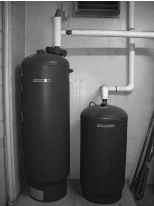
FIGURE 4-25 Photograph of an expansion tank.
