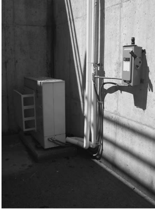
FIGURE 7-12 Photograph of a ductless split-system outdoor unit.
