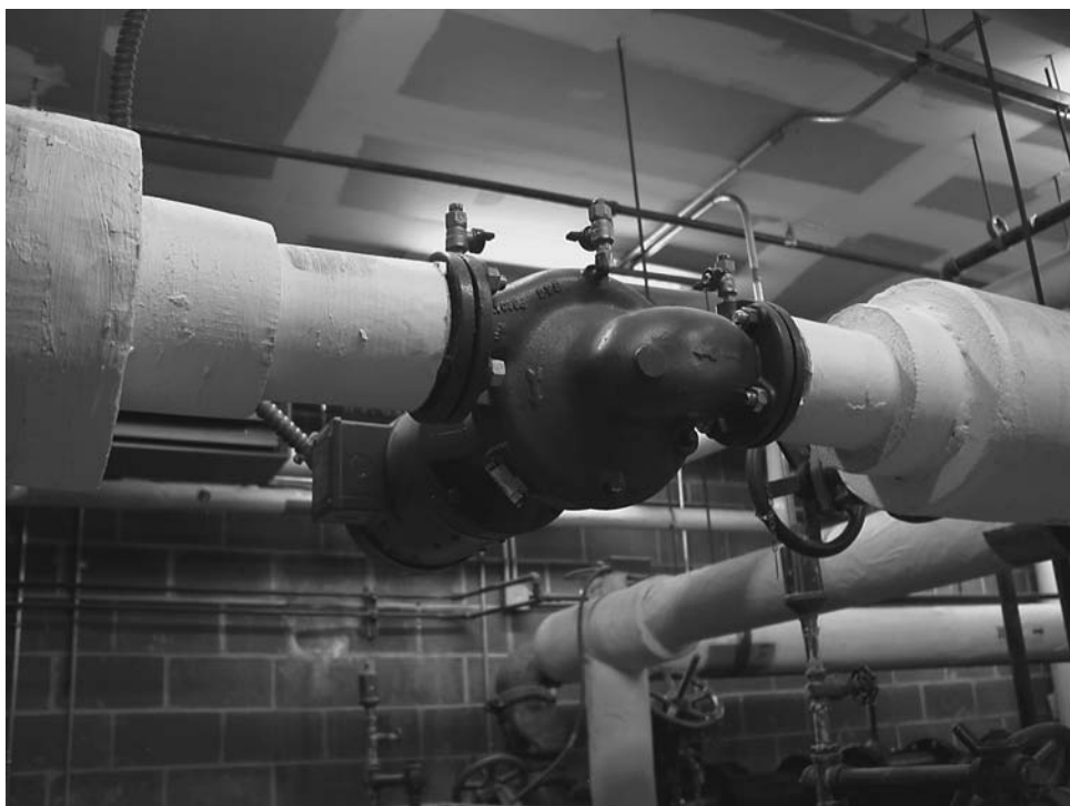
FIGURE 4-33 Photograph of an in-line pump.
