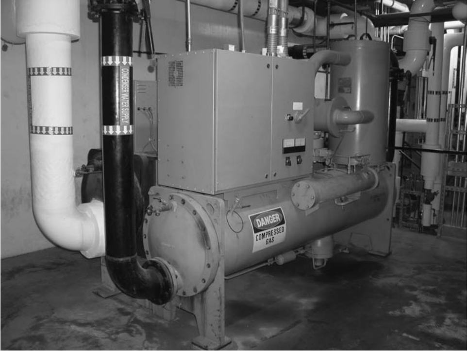
FIGURE 4-12 Photograph of a water-cooled chiller.
