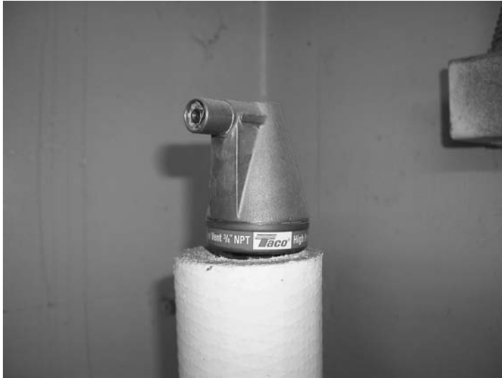
FIGURE 3-40 Photograph of an automatic air vent.
