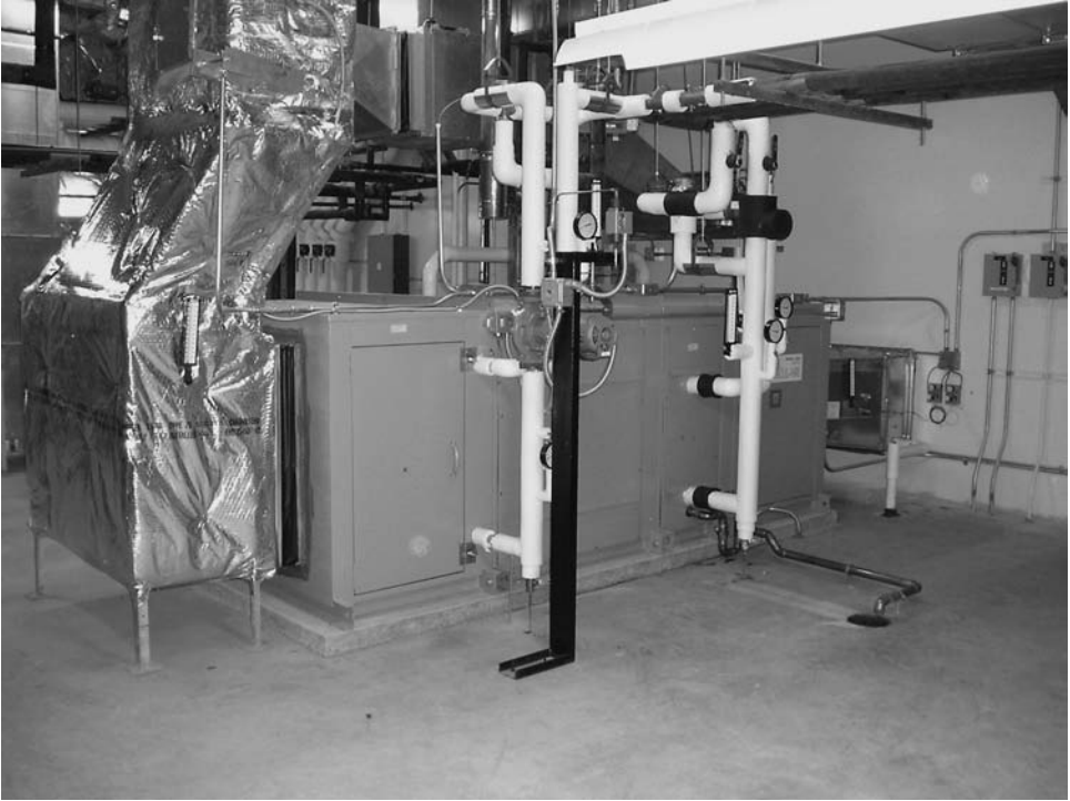
FIGURE 10-6 Photograph of the air handling unit shown in the section drawing (Fig. 10-5).
