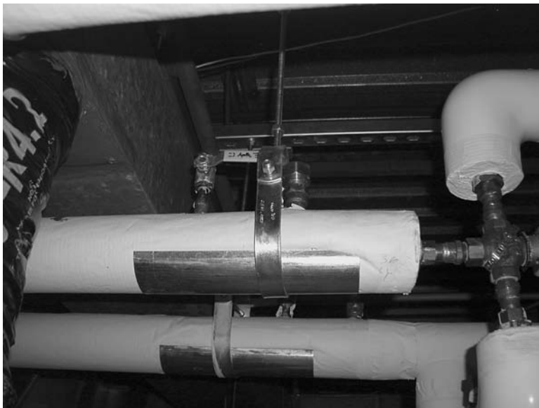
FIGURE 3-34 Photograph of a test plug (the plug is located just to the right of the pipe hanger).
