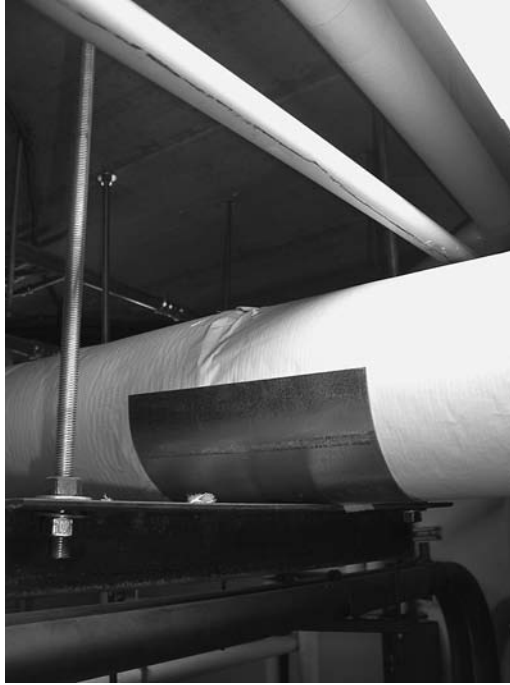
FIGURE 6-4 Photograph of a trapeze pipe hanger.
