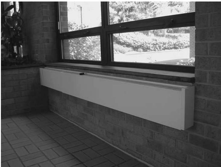
FIGURE 7-4 Photograph of a wall-mounted FTR with manual damper, which controls the airflow through the FTR.
