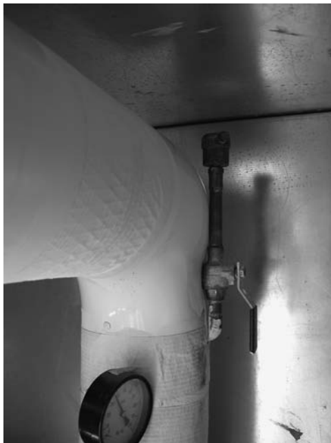
FIGURE 3-39 Photograph of a manual air vent.
