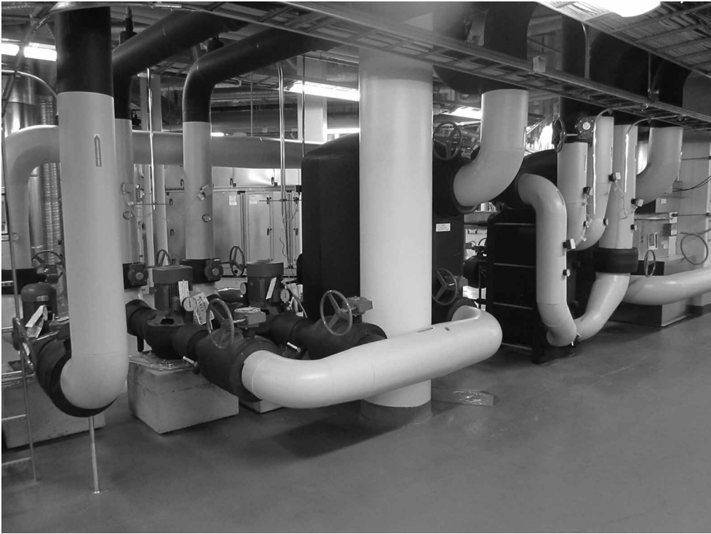
Figure 1. A cooling system in 'triangle-hospital' in Helsinki, Finland.
